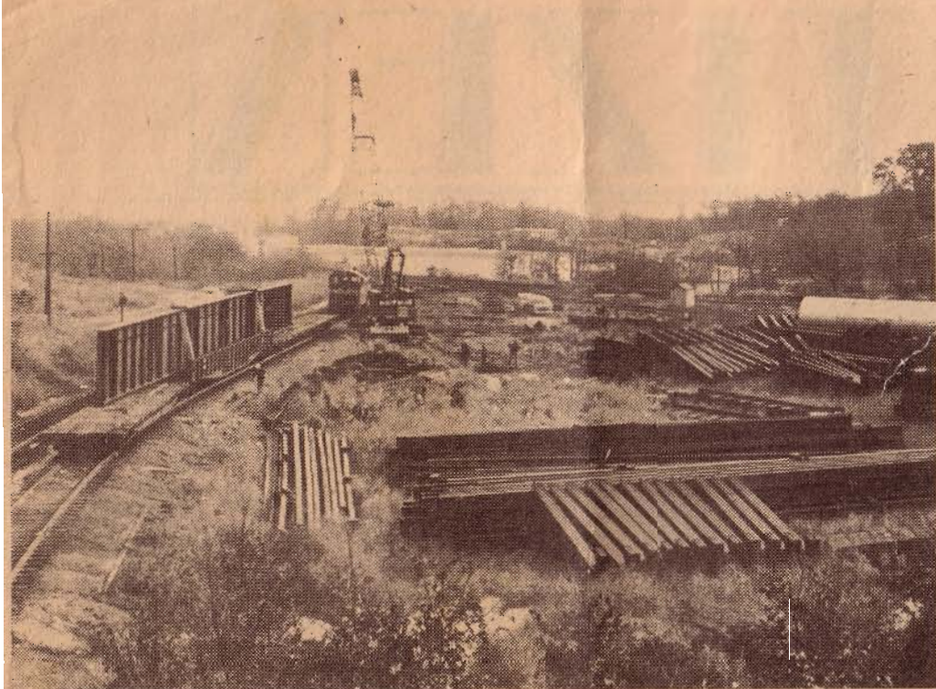
Steel for the construction of an added bridge span to expand the Garden State Parkway crossing of the Raritan River is shown being delivered to the Raritan River Rail-
